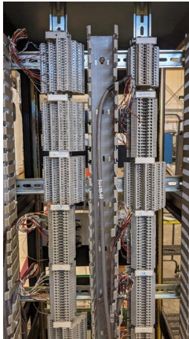
Fig .1. Instrumentation rack #1, rear panel, upper section. Terminal blocks used for PLC IO module connections
